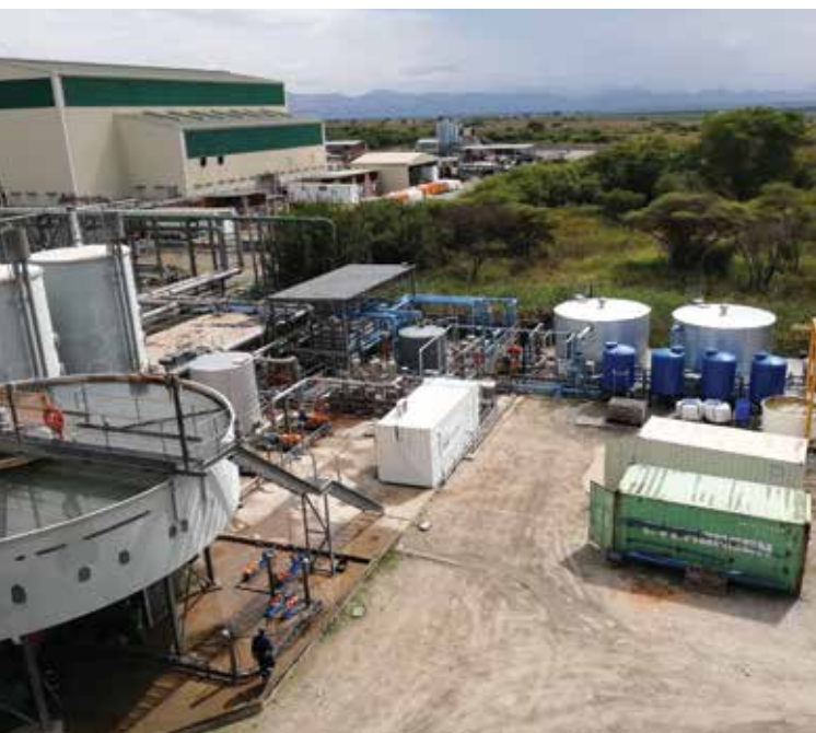
AECI Water treatment plant at Platinum mine in the North-West province. Finalising Phase 2 for treating and reusing a portion of its excess underground fissure water to reduce potable water consumption results in significant cost savings but also contributes to the continued sustainability of mining operations and the community.
