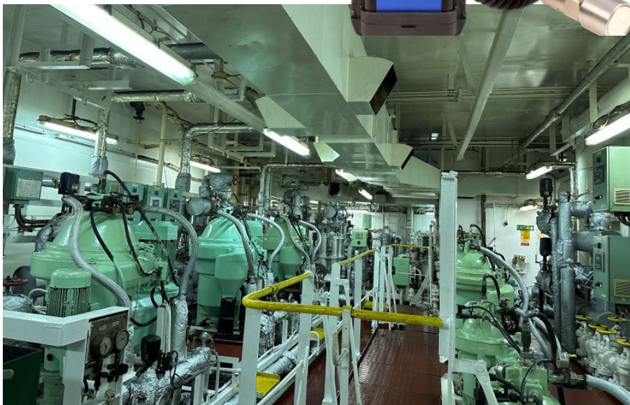
AN ON-GOING MONITORING STRATEGY IS CRUCIAL TO MAINTAINING THE SERVICE LIFE OF ROTATING EQUIPMENT, TROUBLESHOOTING PROBLEMS, AND PREVENTING FAILURES, AND SUBSEQUENT COSTS
